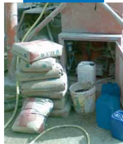
Mechanical system for metering Mapescreed 704
